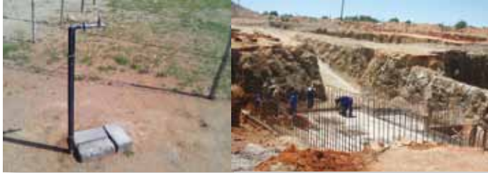
Water and sanitation provision
