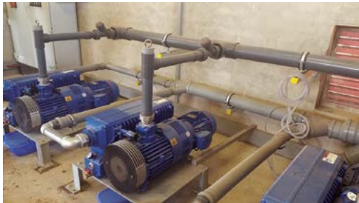
Pumps in vacuum station
