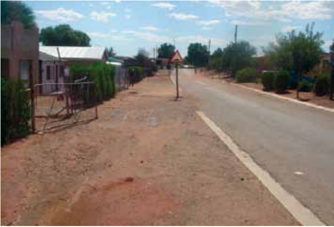
The floor levels of these houses are much lower than the finish level of the road
