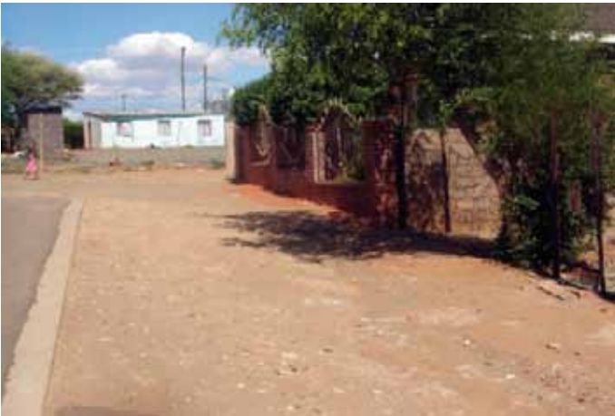
Erosion because of stormwater drainage problem
