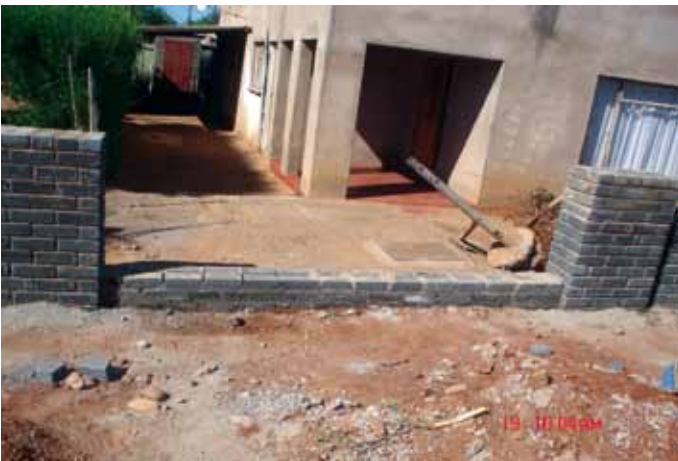
Preparation work to lay paving. Laying of foundation for the construction of retaining wall.
